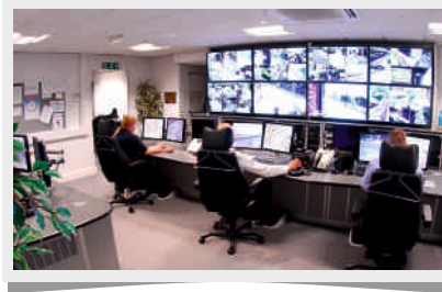
SECURITY AND SURVEILLANCE
